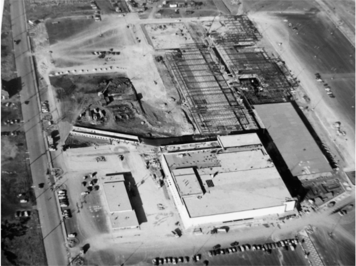
The Polo Park site while under construction Photo from Old Manitoba, The Way It Once Was!
