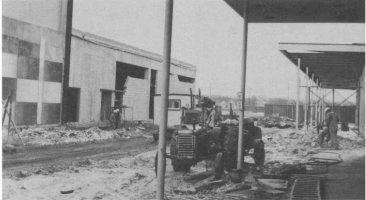
Construction crews dig the foundations of Eaton's court From Retro St. James
