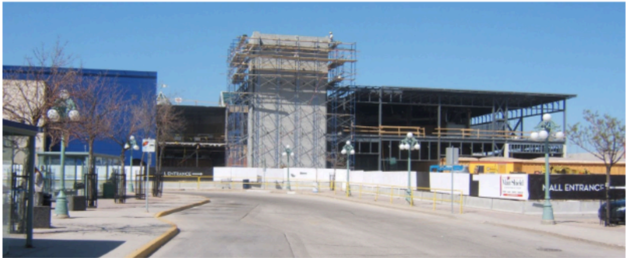
South Entrance under redevelopment in early 2007. Photo from CF Polo Park archives.
