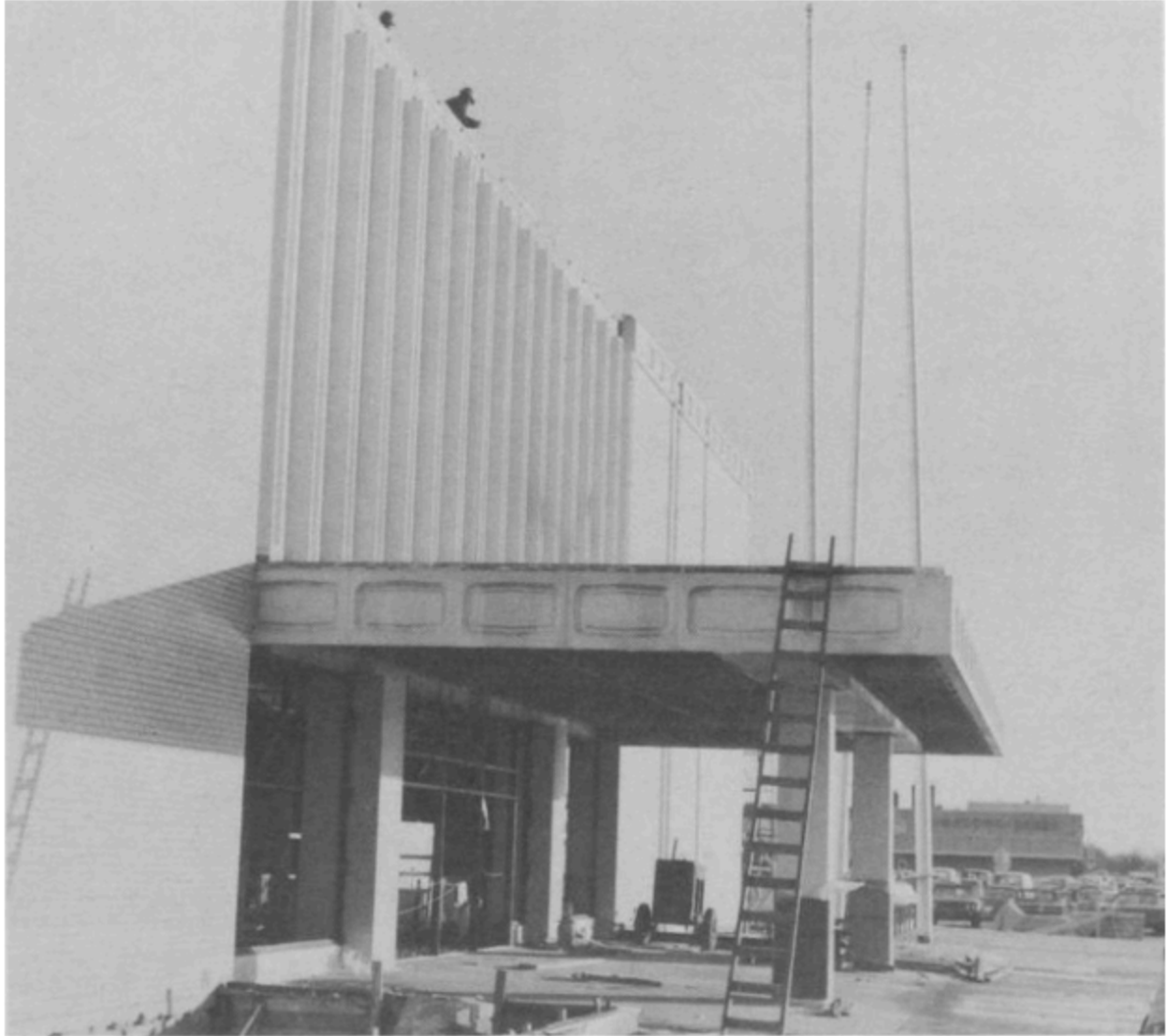
Construction of the new Eaton's building at the north end of the mall. Photos from Retro St. James
