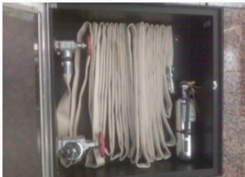
75–100 ft. of fire hose/10 lb. ABC Multipurpose extinguisher
