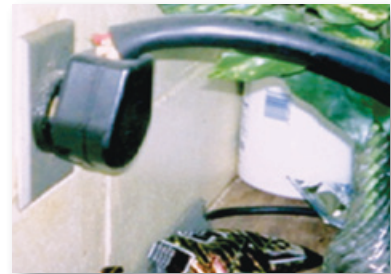
Frayed Electrical Connection
